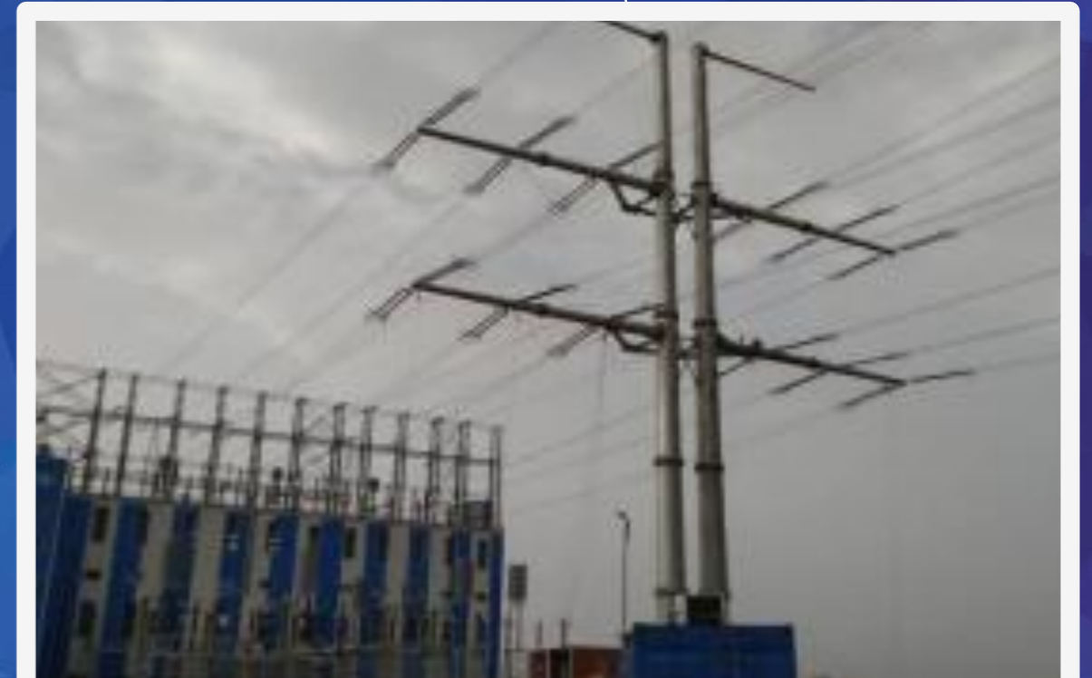
Transmission Line Monopole
