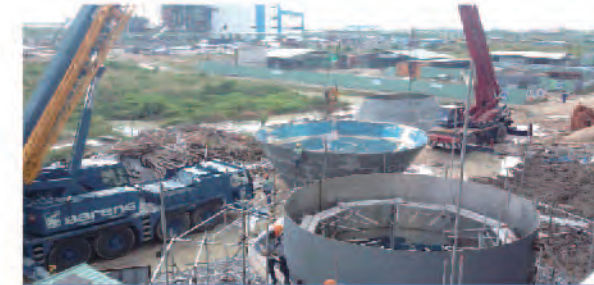
不锈钢SUS304+Q345R复合板-正隆纸浆储罐 Supplied SS SUS304+Q345R Clad Plates for CHEN LOONG Paper & Pulp Storage Tank
