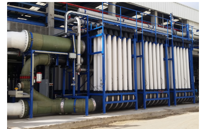
Industrial Waste Water Treatment
