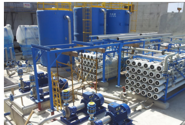
Industrial Water Treatment
