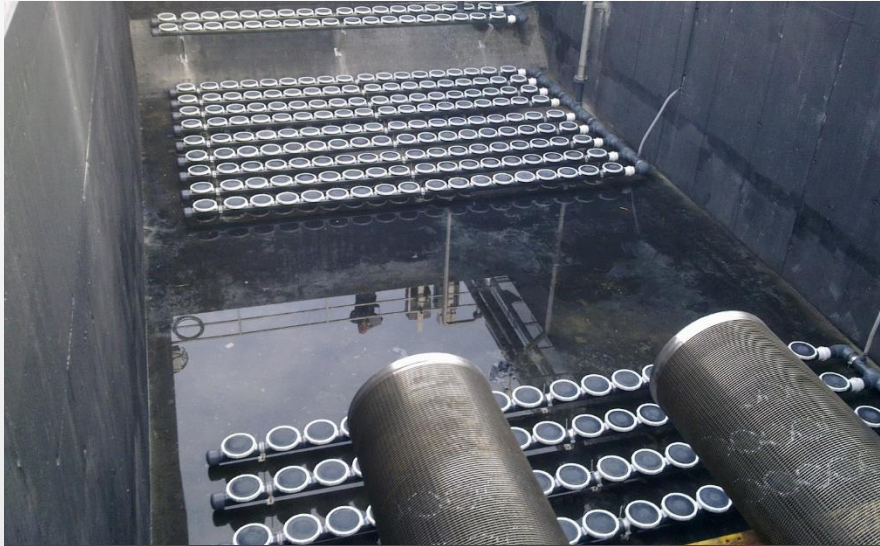
Gambolo WWTP, Italy
