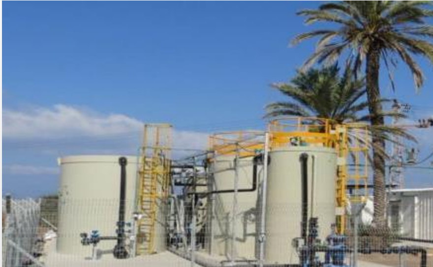
Ground Water Treatment - Sdot Yam, Israel
